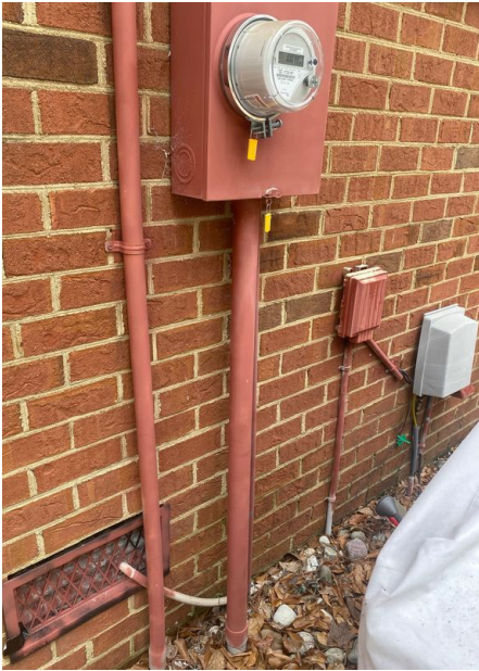
Service Equipment/Electrical Panel: Electrical Panel / Service Equipment Location Kitchen
